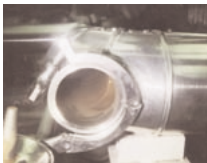
Fig 2. Rouging in a WFI pipe arrangement.
