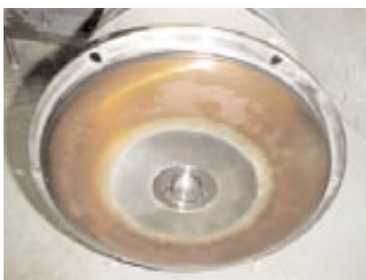
Fig 3. Rouging in a WFI pump.
